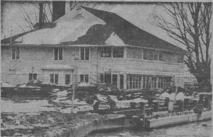
GOING UP —To escape high water, Rochester Yacht Club building in Summerville is being raised 3 feet.
