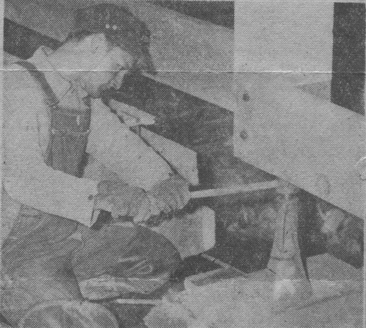
HERE'S HOW —Jerry Williams, 61 Castleford Rd., Greece, operates one of the jacks used to hoist clubhouse.
